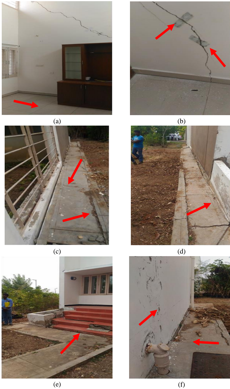
Fig.1 (a) View of caving-in of vitrified tiles and (b) diagonal wall cracks in the inner portion living room area; (c),(d) Caving-in of the plinth protection slab southern side (e) Damages of platform and footstep of eastern portion of the building (f) Views of wall crack and caving-in of plinth protection slab on northern side
